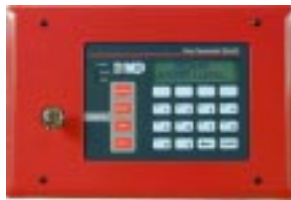
Fire Command Center
